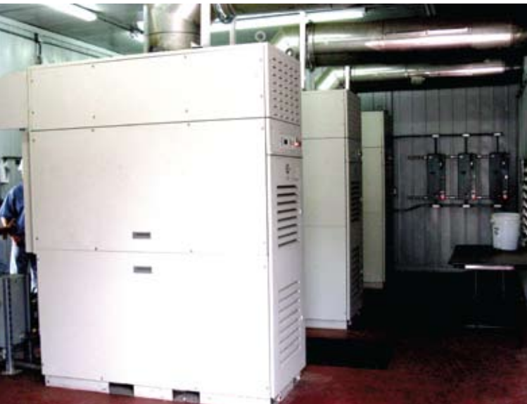
Three Capstone C65 ICHP microturbines operate on the pipeline natural gas that's pumped through Crayne Station. Heat exchangers on the top of each microturbine capture waste heat used in the decompression process.
