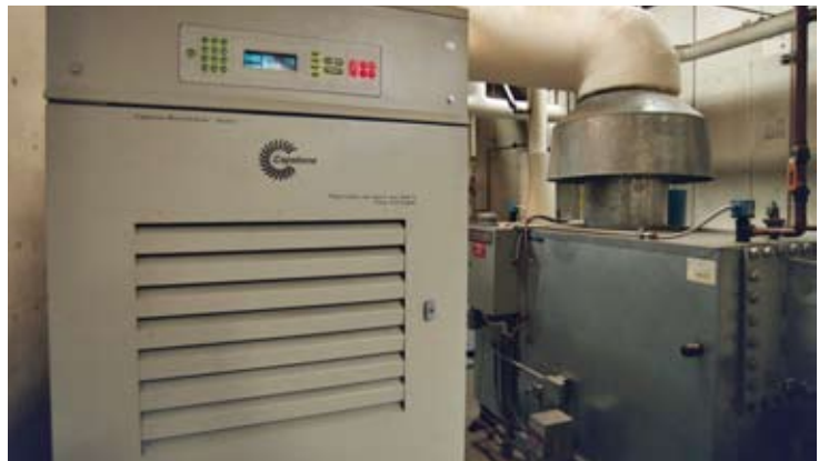
A Capstone microturbine provides electricity, cooling and heating to Citibank in La Jolla.
